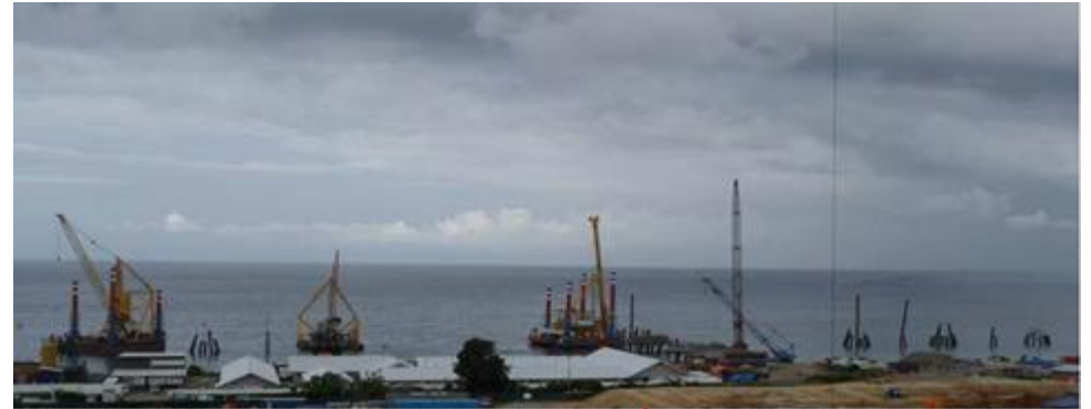
F100: LNG Jetty Area - Piling works on Trestle & Jetty Head in progress - Headstock concrete work for trestle in progress.
