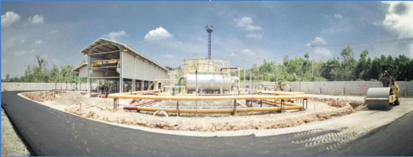
View of EOR Station from SP Injection & Production Area
