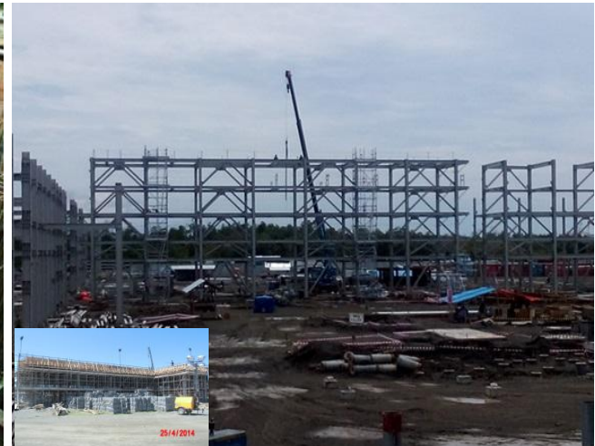
Main Pipe rack
