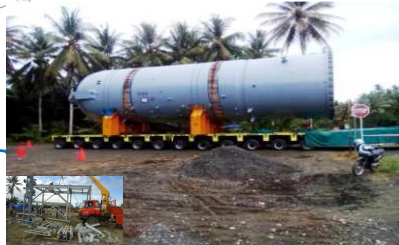
H2S Removal vessel
