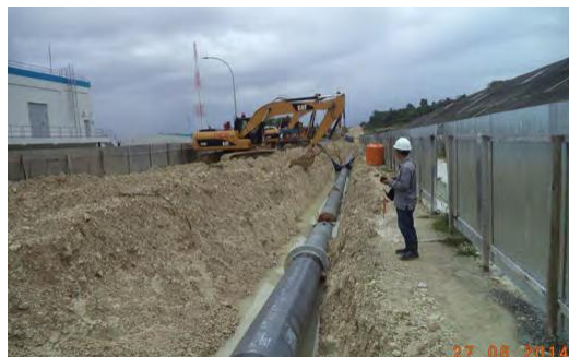
Anchor Flange at KP 23+000
