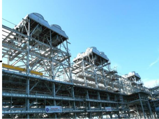
Air Cooler Installed at Main Rack
