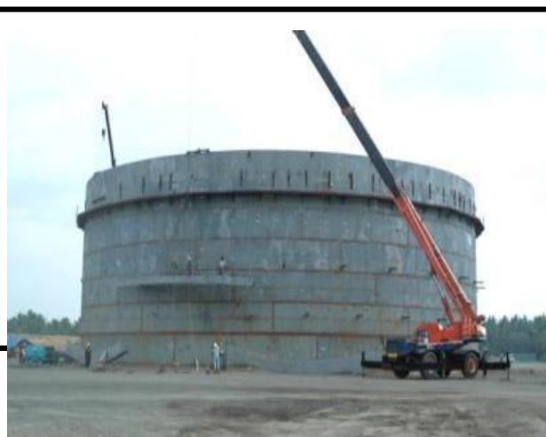
Condensate Loading Tank
