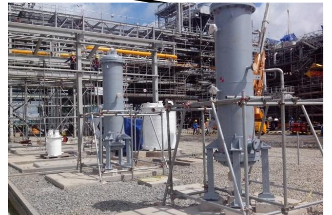
Water Treatment Installation
