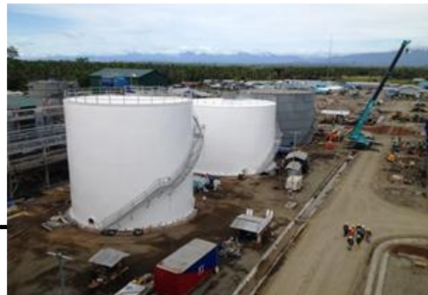
Condensate Loading Tank
